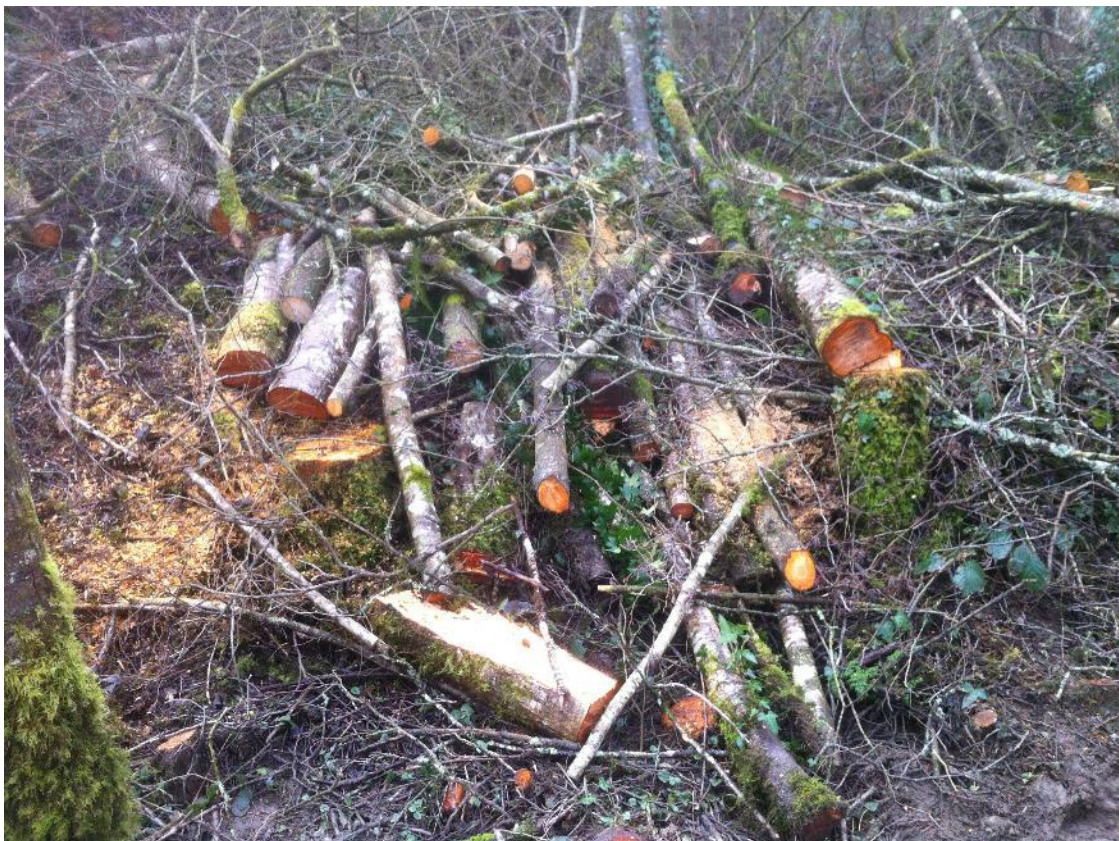
Figure 4 Trees cut down in the process of Action C5 were stockpiled and used to construct log piles for Action C7
